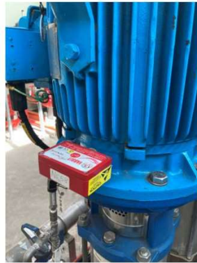
Pump monitoring using IoT
